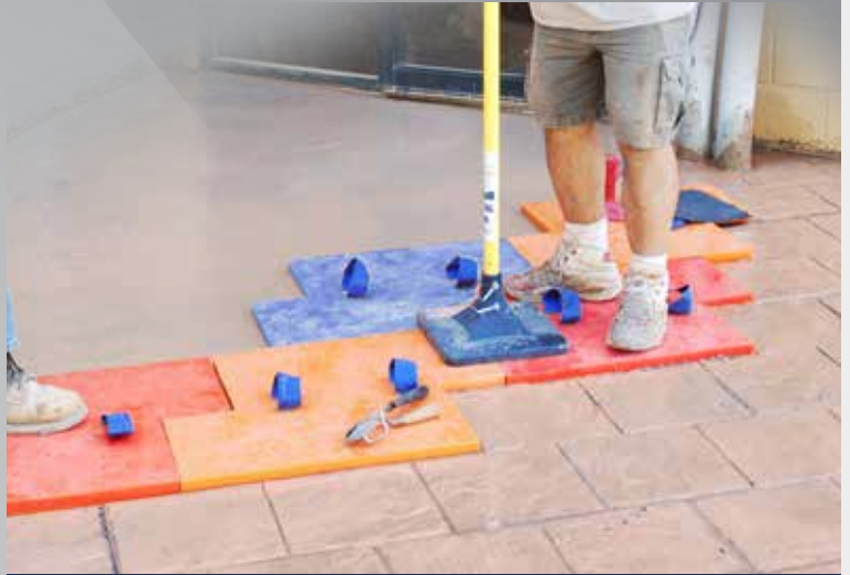
8 Stamps are positioned and hand-tamped to imprint the pattern on the concrete slab.
