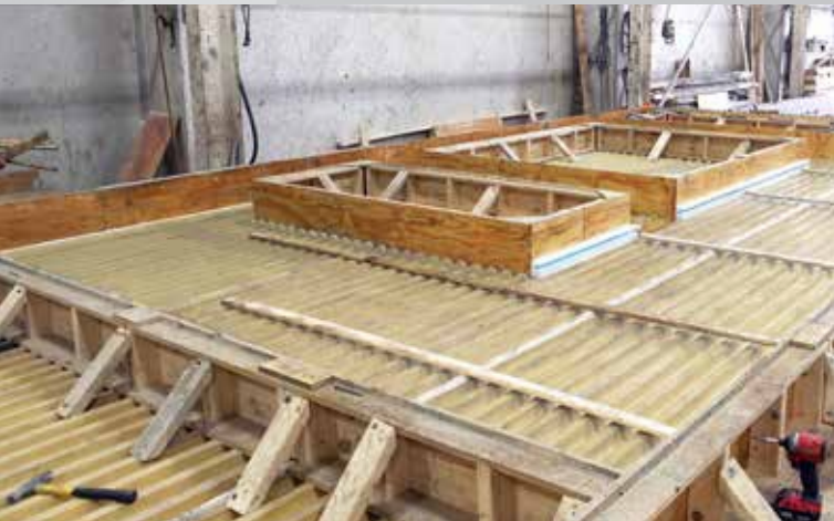
5 VytaFlex™ liners are positioned on the casting deck. Form walls are built around the perimeter and for window knockouts.
