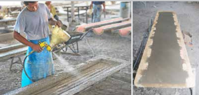
7 A face coat of GFRG is sprayed onto the mold surface using a hopper gun followed by a base pour of concrete and chopped glass. The mix is allowed to cure.
