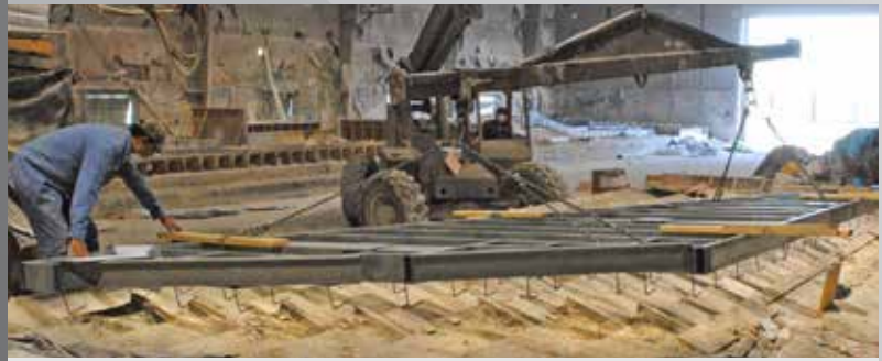
5 A structural steel frame is carefully lowered into place just above the wet concrete.
