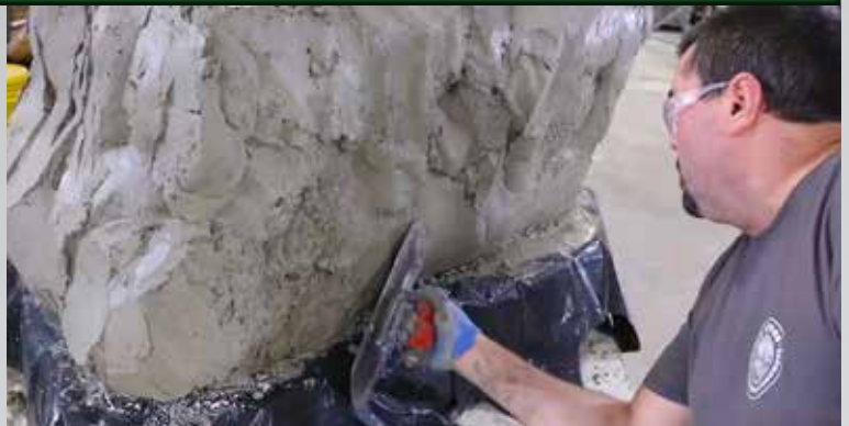
8 The surface layer of Vertical Mix™ is applied, and roughly carved and shaped to imitate stone.
