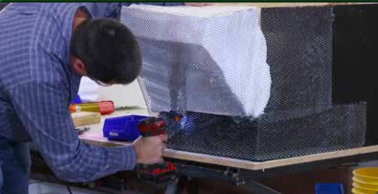
7 Foam and metal lath are attached to a wooden base to create the rough shape.
