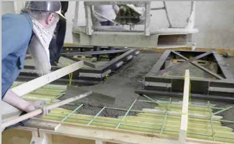
6 Rebar is positioned over the form and concrete is cast. A layer of insulation is sandwiched between two layers of reinforced concrete.
