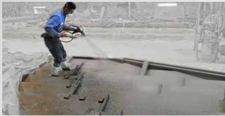
2 Additional layers of backup mix reinforced with AR glass fiber are applied.
