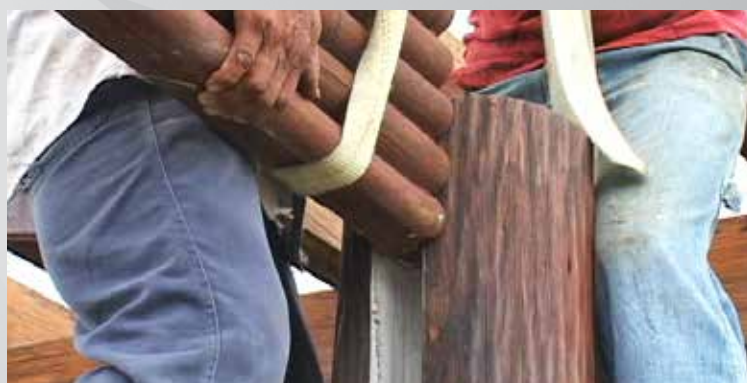
12 Once cured, artisans align lightweight GFRG bamboo panels with pre-fabricated channels in the columns which makes placement easy.
